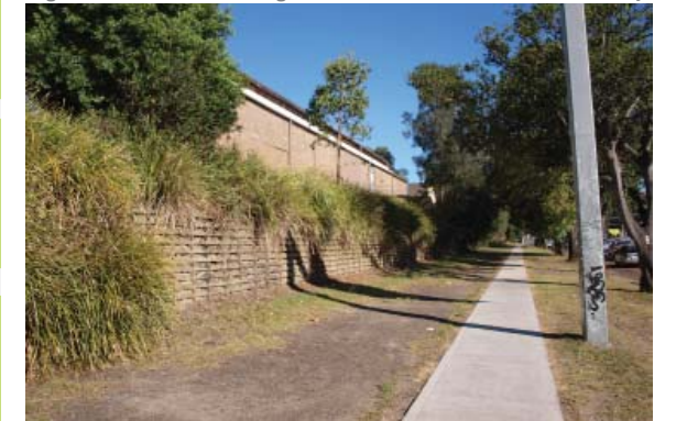
Figure_1.53. Retaining wall along Anzac Parade creating a barrier to E.S. Marks Field
